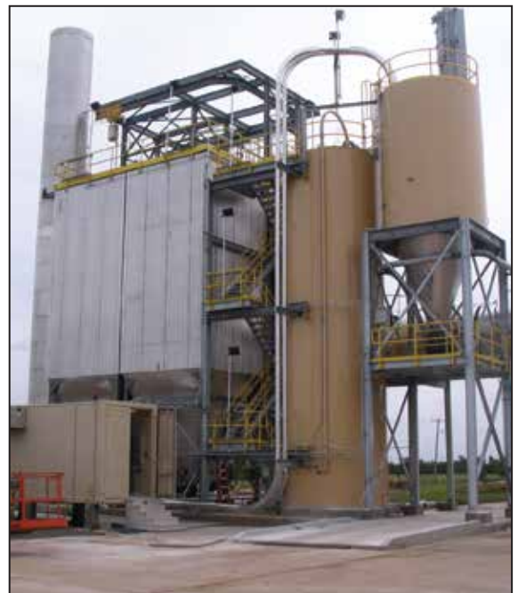
Fabric Filter with Dry Sorbent Injection on a Brick Kiln
