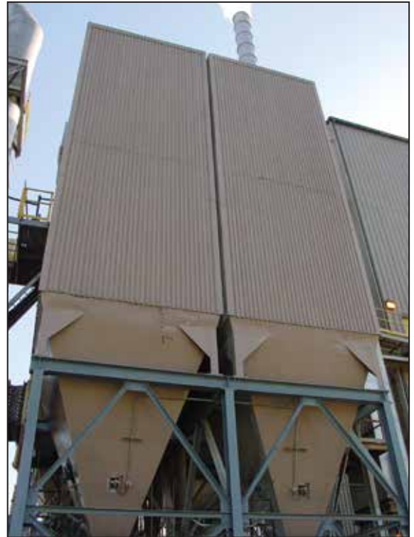
Fabric Filter as Part of a Circulating Dry Scrubber on a Specialty Metals Application
