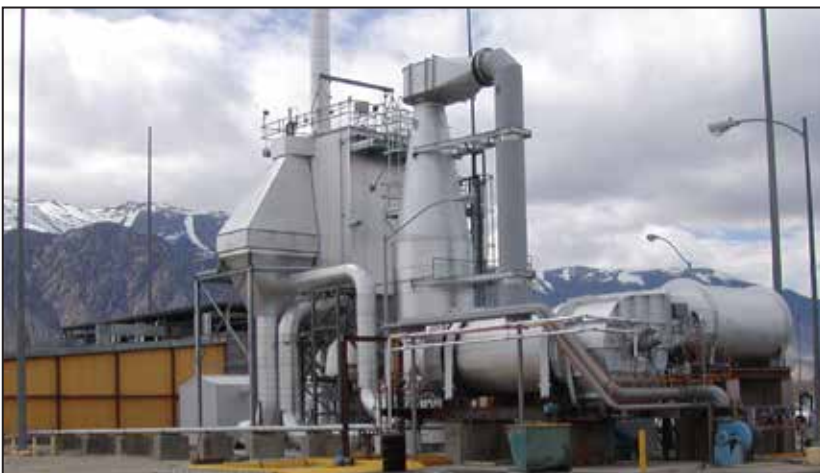
Fabric Filter with Dry Sorbent Injection on a Military Propellants Incinerator
